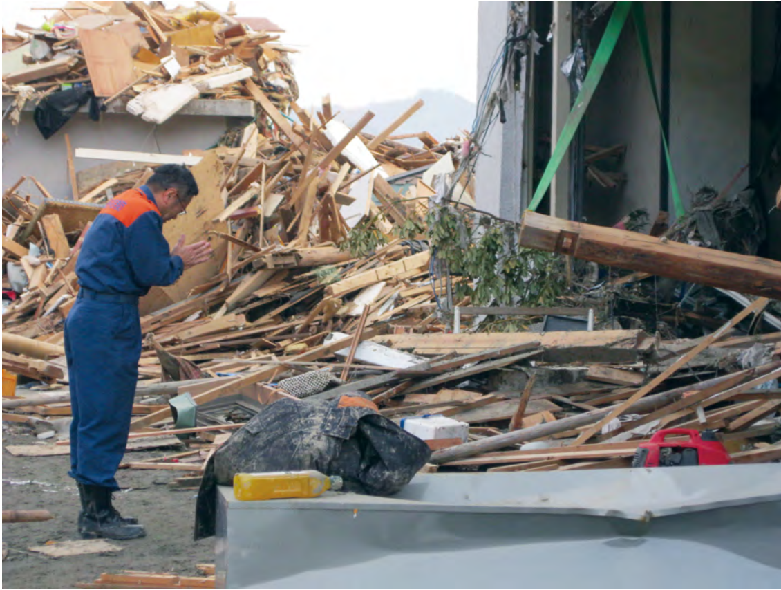
▲ Then chief of the fire station holding his hands in prayer in front of the completely destroyed fire station
