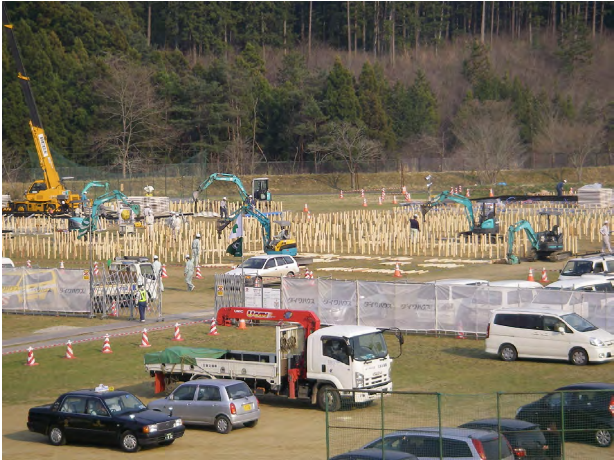
▲ Construction of temporary housing commencing in the school grounds of Shizugawa Junior High School
