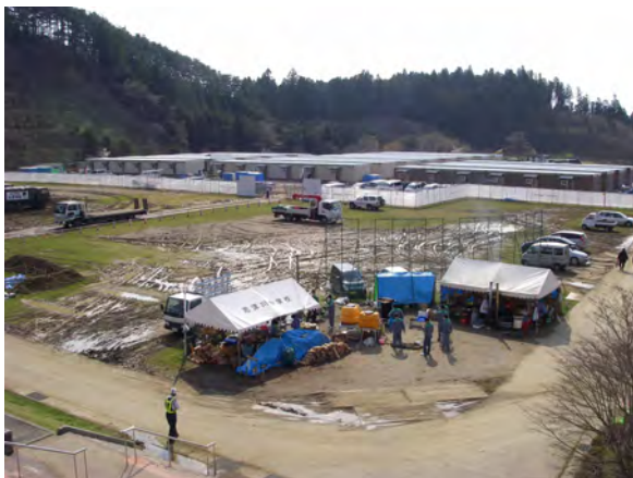
▲ Temporary housing complex under construction in the school grounds of Shizugawa Junior High School
